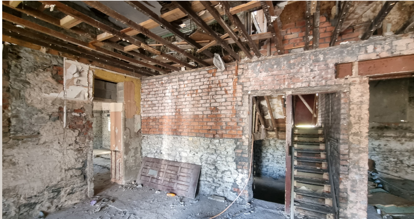
► Image 9: Indication of the current dilapidated `state` of the existing building with partially completed works
